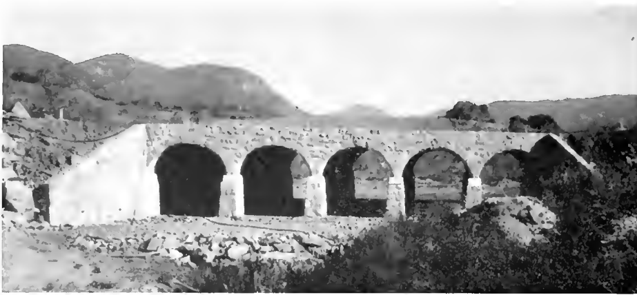
FIG. 57. Quintuple culvert of rubble masonry and metal arches, Moosa Canyon on State Highway in San Diego County
